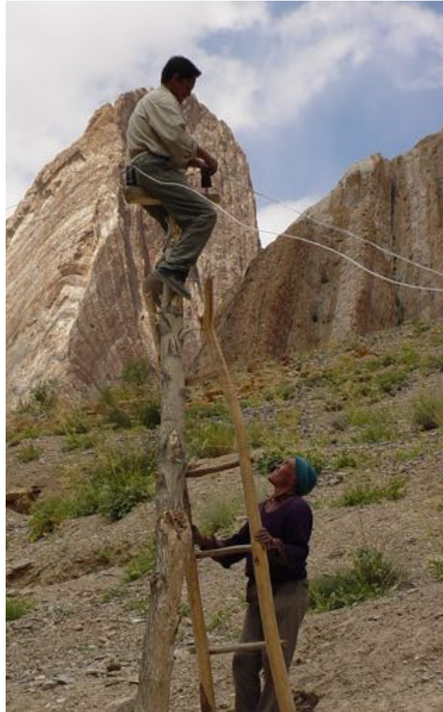
Micro-hydro transmission line being installed by the Ladakh Ecological Development Group (LEDeG) with Honupatta villager in Ladakh, India. Photo by Dipti Vaghela.
